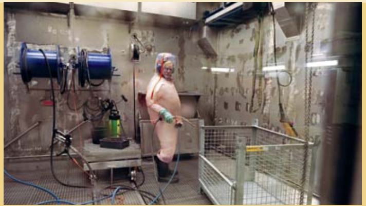
Components being cleaned in the wet box of the Siempelkamp decontamination cell
