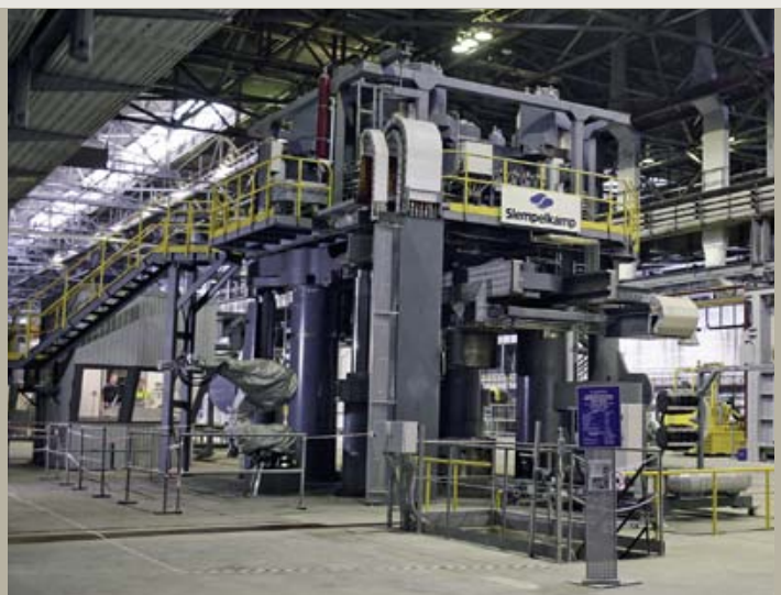
20,000 t press ready to start operation
