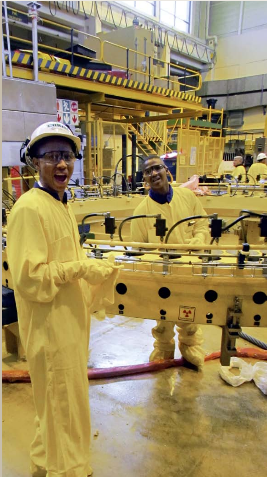
The multi-stud tensioning machine at the Koeberg nuclear power plant, South Africa
