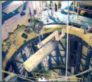
The main coolant lines being drawn out of a device of the biological shield for dismantling
