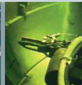
Dismantling of the thermal shield using the plasma cutting process under water
