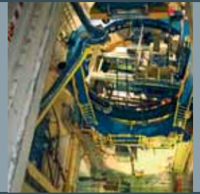
The dismantling of the RPV and its installations is followed by the dismantling of the equipment and decontamination of the rooms
