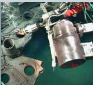
Application of the thermal and mechanical dismantling process for the moderator tank under water
