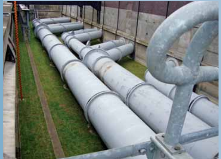
Pipeline supplies to the turbine house
