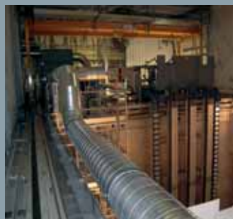
Installed ventilation technology
