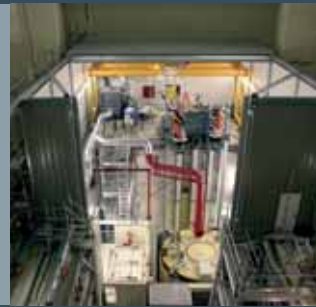
View of the ventilation technology housing over the fuel assembly storage pool – set up for dismantling
