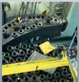
Dismantling of the RPV lid and the packed bed using a mobile band saw in the air
