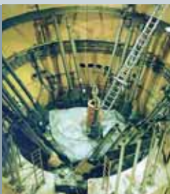
Initial situation: view of the RPV before the start of assembly and dismantling
