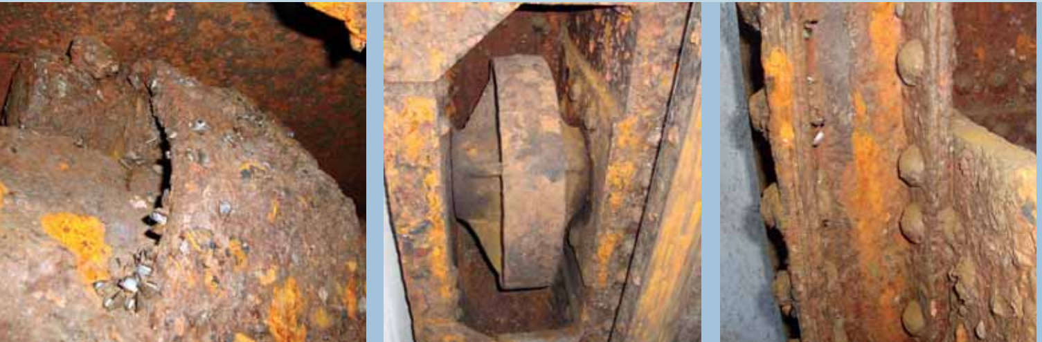
Severe plate rust and shell deposits on pumped-storage power plant components: fastening element, guide roller and rivet connection of section and sheet
