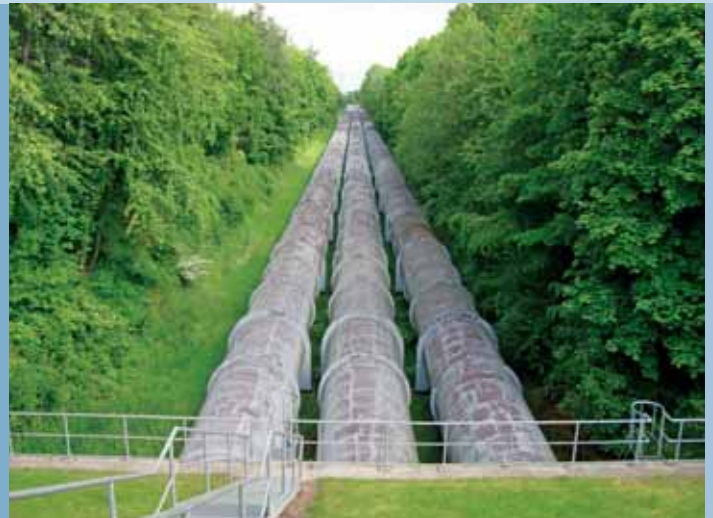
Valley-side pipelines on the Niederwartha pumped-storage power plant
