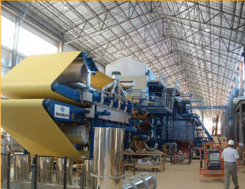
Huber ContiRoll® and preheater during assembly
