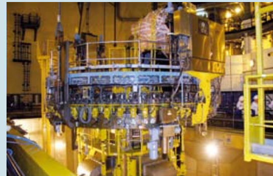
Stud tensioner at the nuclear power plant Cattenom
