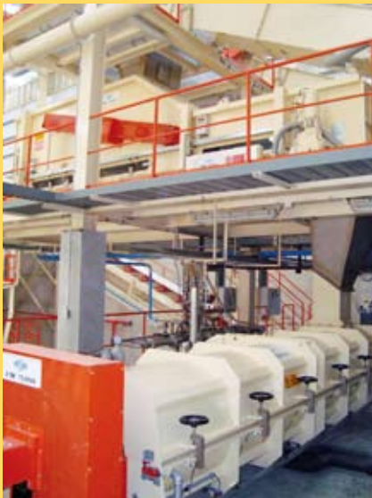
Dry particle silo and resin blender
