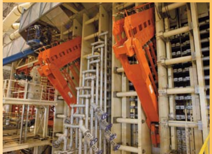
Canfor-LP multi-daylight press after completion
