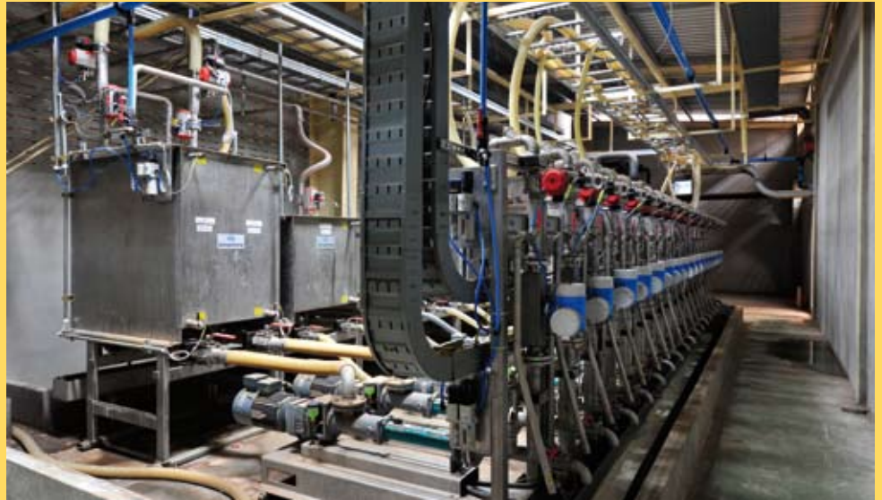
Glue kitchen with dosing system
