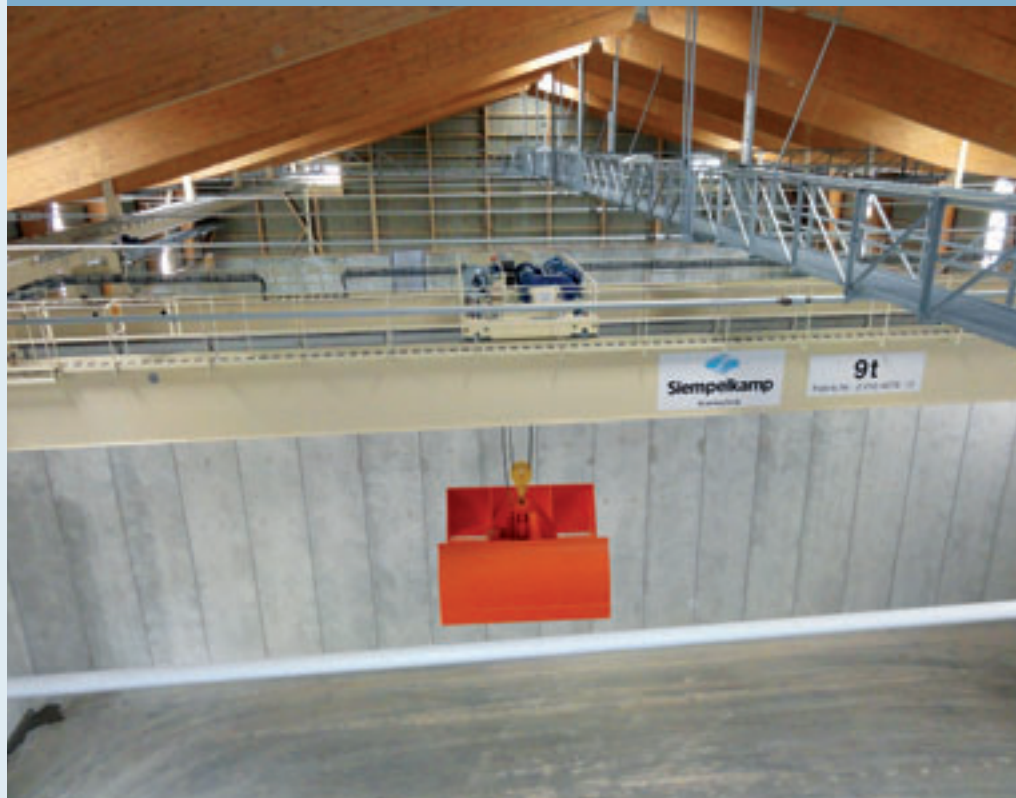
Fully-automatic suspension crane system with grab fully assembled inside the depot
