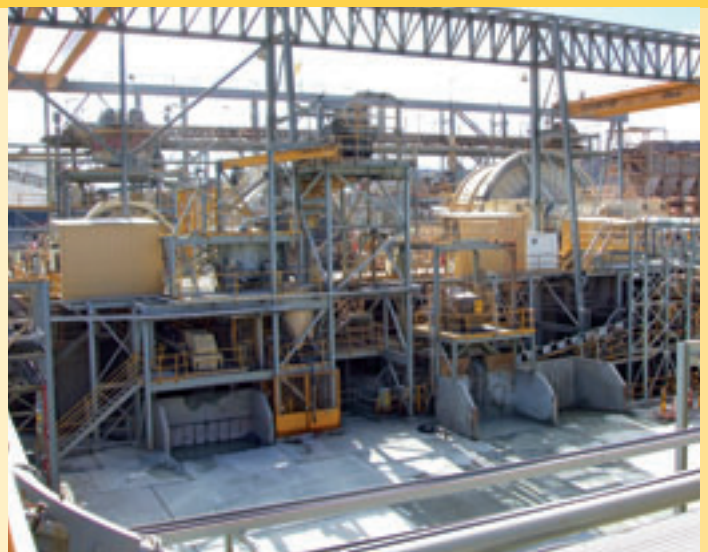
Complete system for the grinding process of rocks at the copper
